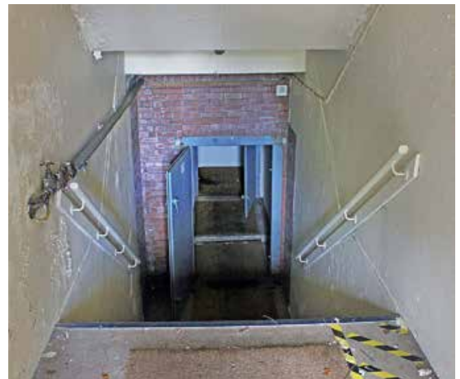
View from main entrance looking down access stairs. This connection was formed as part of the 1980's alterations
